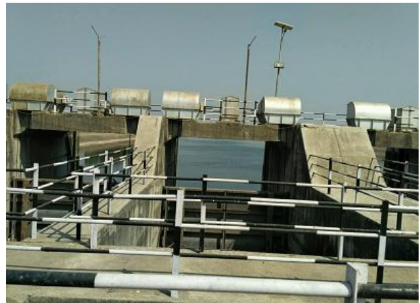
Motors installed for controlling Gate operation at Sabarmati Canal Syphon
